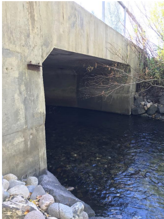
Photo 3. Looking downstream face of SH-75 Bridge over Trail Creek from right bank on October 8, 2019.
