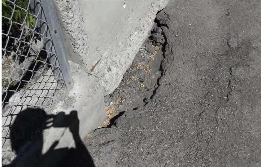
Erosion under rail at northwest corner
