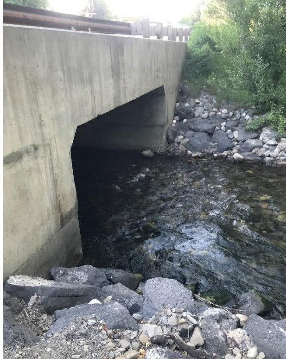
Photo 2. Looking upstream face of SH-75 Bridge over Trail Creek from left bank on July 28, 2019.
