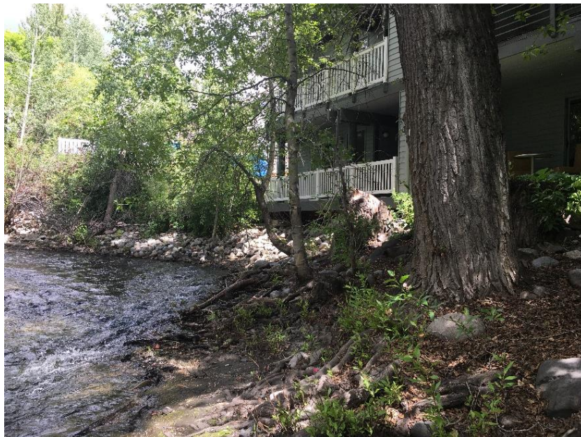
Photo 8. Bank Protection and Tree Roots along the left (south) bank of Trail Creek Upstream of SH-75 Bridge
